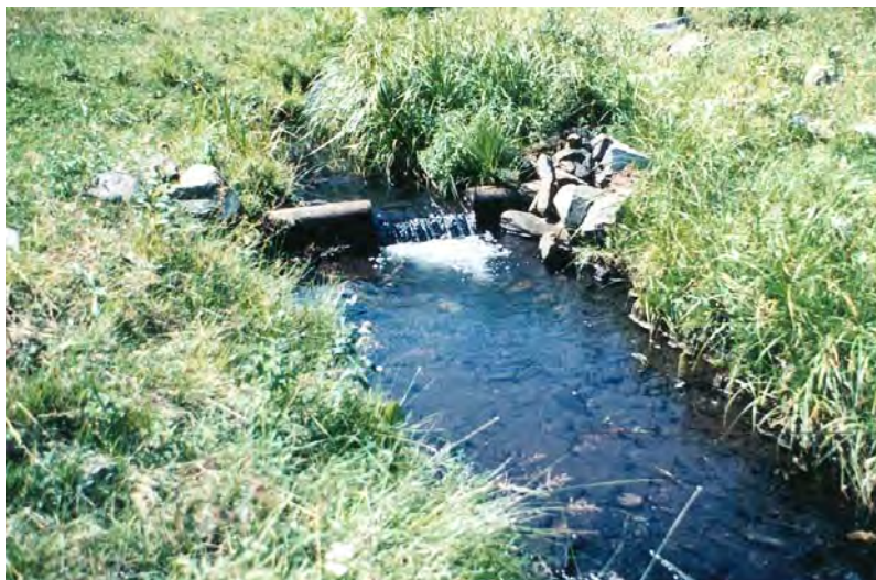
Figure 59-2. Building timber plunges in Spotted Tail Creek created deep plunge pools, and in some cases, dam pools. An additional benefit was increased sub-irrigation of the riparian area as the plunges raised water tables in the floodplain.
