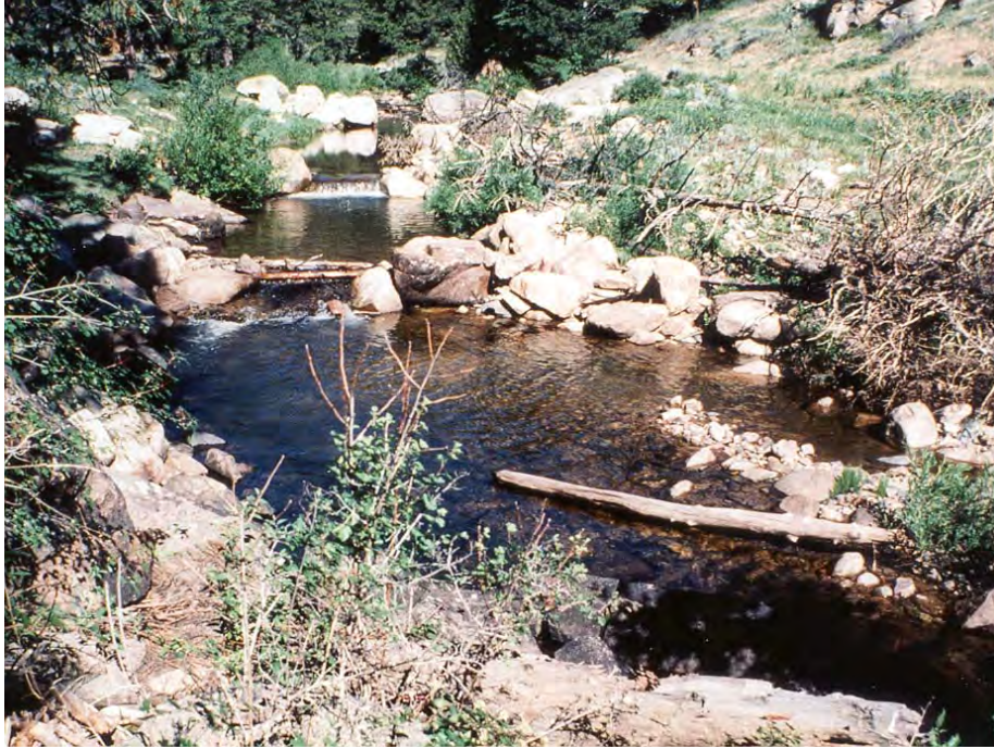
Figure 30-5. A pair of boulder plunges (foreground) and a boulder double deflector (top of photo) as they appeared soon after construction.
