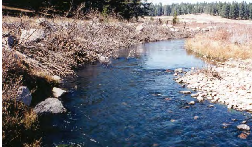
Figure 27-2. Larger conifers and less rock were used in this revetment, seen here three years posttreatment.
