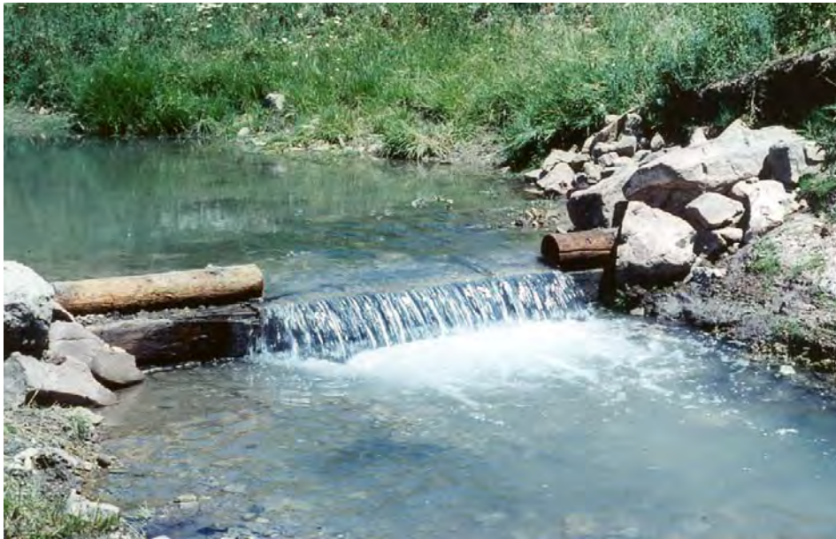
Figure 13-2. A freshly installed timber plunge in Coal Creek already provides pool habitat to shelter trout.
