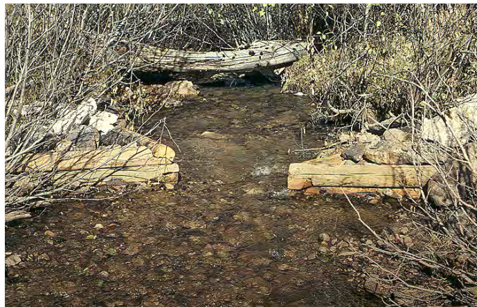
Figure 48-2. Double deflectors were installed in Pass Creek to narrow the stream flow and encourage scouring of pools for trout shelter.
