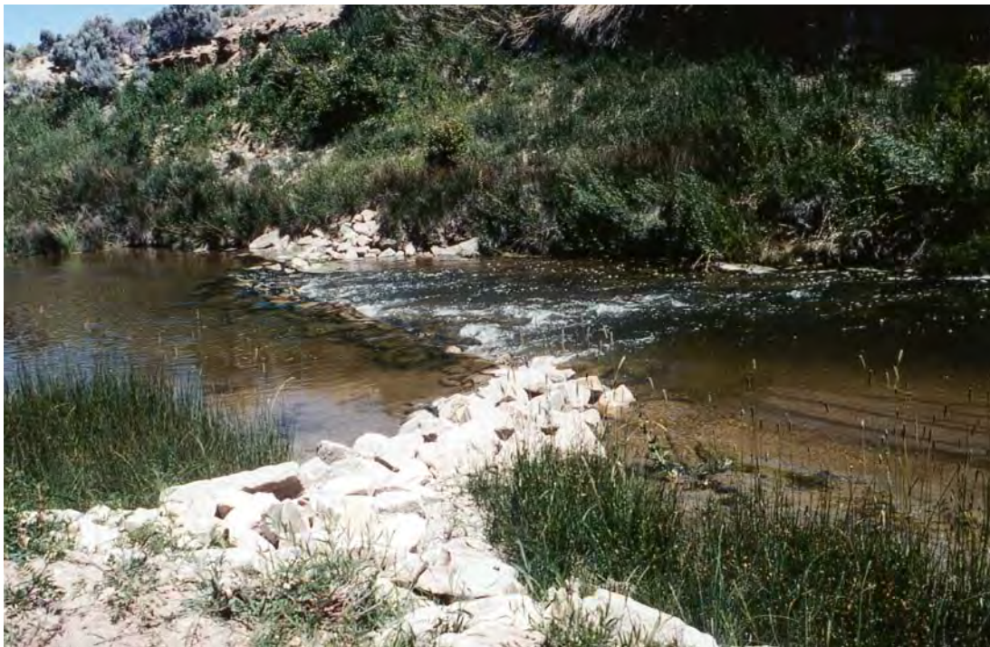
Figure 6-1. Addition of rock weirs to the Big Sandy River increased habitat diversity by creating dam pools, plunge pools, and turbulence. Spaces between the rocks are important shelter for juvenile trout. These weirs also acted as grade controls and raised the local water table, which better subirrigated riparian vegetation near the weirs. The stream narrowed as sediment deposited in new lateral and point bars and riparian vegetation colonized these bars.
