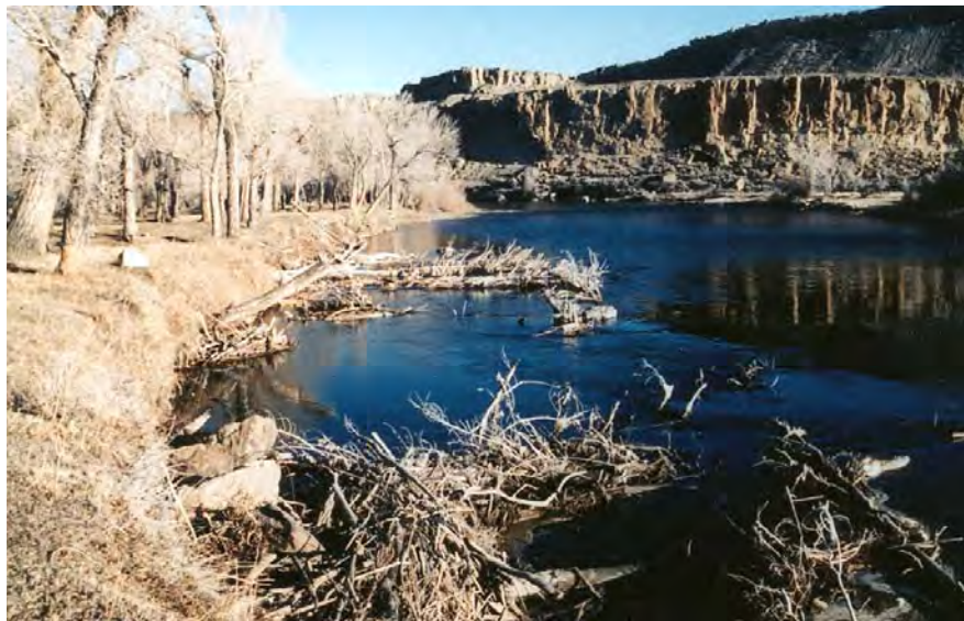
Figure 46-1. Tree jams were constructed in the North Platte River at Pick Bridge as an experiment to determine if this type of structure was feasible for this river.
