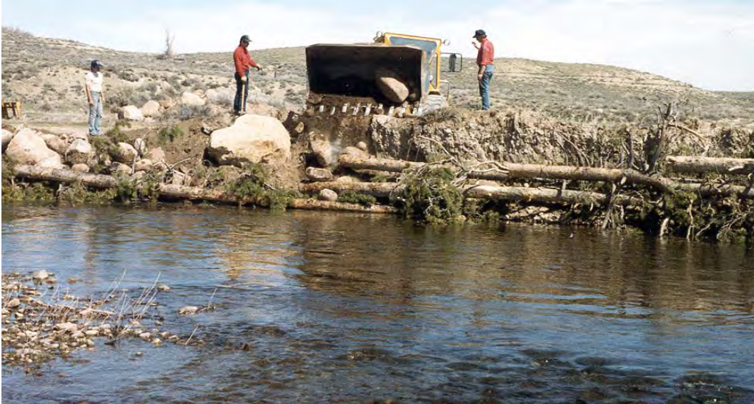
Figure 41-2. A construction crew adds rock riprap behind tree revetments at the PFA on the North Fork Popo Agie River.
