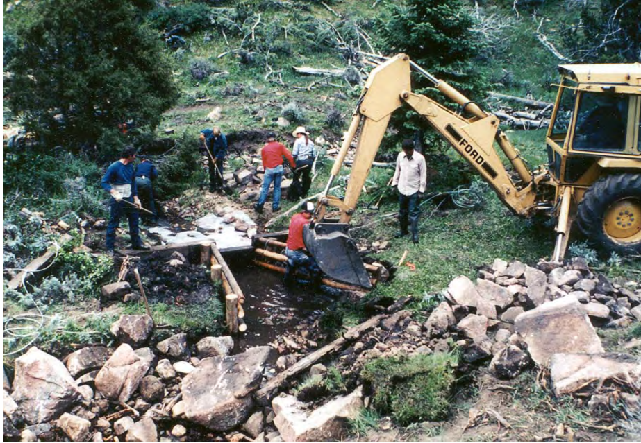
Figure 24-2. A joint WGF and USFS work crew building a timber plunge in 1985 to provide deep pool shelter for trout in the rocky substrate at Hall Creek.
