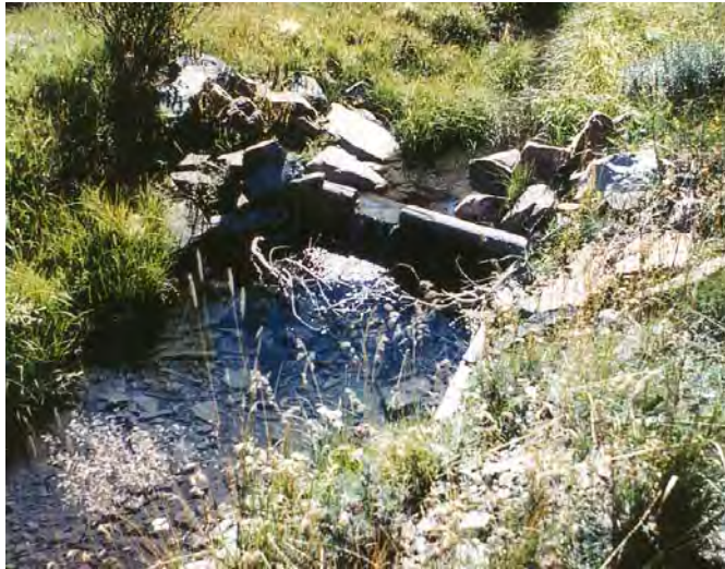
Figure 40-3. A close-up view of a timber plunge in Nameless Creek.
