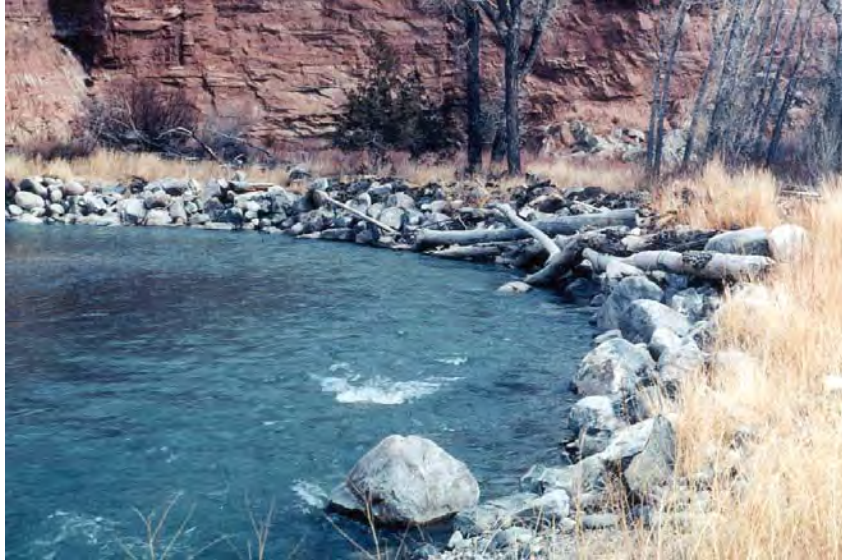
Figure 66-1. A formerly eroding stream bank has been stabilized with rock riprap. Woody debris visible in the picture washed in naturally during floods.
