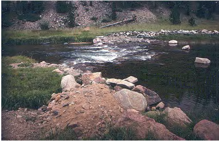
Figure 58-2. Where long shallow runs were present at Shutts Flat, as in Figure 58-1, several rock vortex weirs were constructed to provide deep pool shelter for trout. In addition to providing pools, these weirs act as grade controls and encourage sub-irrigation of downstream riparian vegetation by raising water tables in the floodplain.
