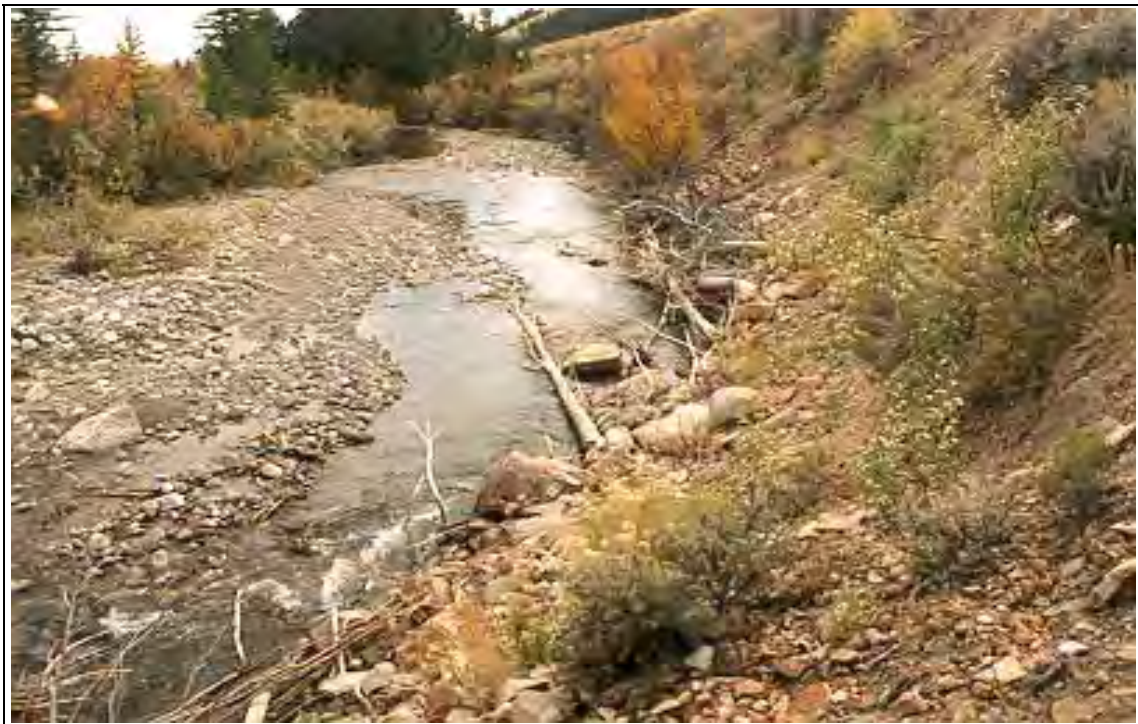
Figure 1-3. Six years after tree and rock revetment installation, severe bank erosion is controlled and the bank is stable. There is good growth and development of plants.
