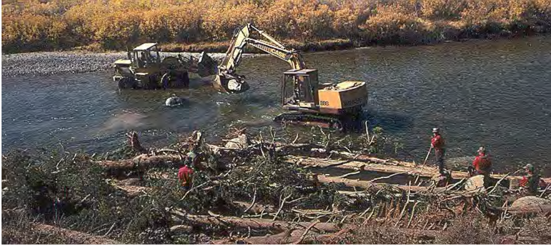
Figure 2. Installation of tree jams on the upper Green River was done with the aid of heavy equipment rented from private contractors. A work crew installed cables after the trees and rocks were placed by the tracked hoe.
