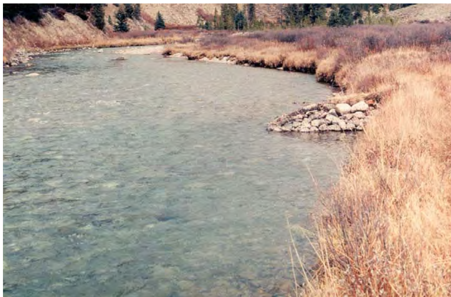
Figure 19-2. A stream-lined wire crib deflector on the south bank of Granite Creek was still largely intact and functional in 1980. A pool/run is present downstream from the point of the device. A similar device on the opposite bank had largely disintegrated by 1980, but the two structures have narrowed the stream at this point. Flow is from top to bottom.
