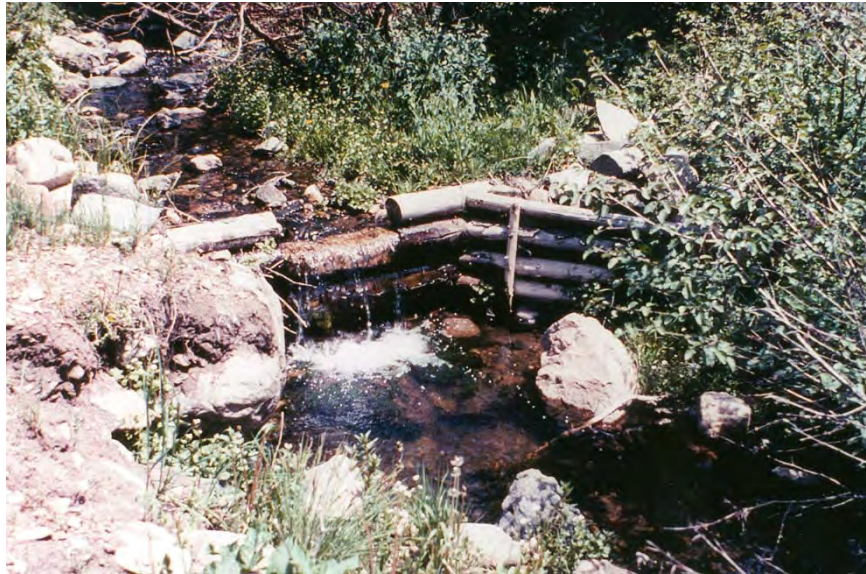
Figure 26-1. A log plunge in Hell Canyon Creek near the forest boundary 14 years after construction is still intact and acting as a grade control. Its plunge pool furnishes shelter to trout and a jumping point for trout seeking to move upstream past the structure.
