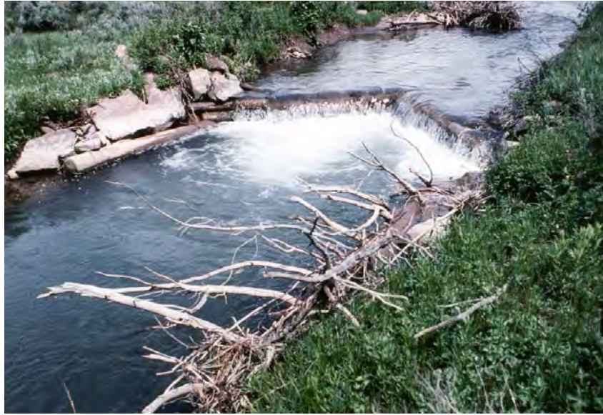
Figure 52-4. A deep plunge pool developed at this upstream “V” log plunge, furnishing valuable deep water cover for trout.
