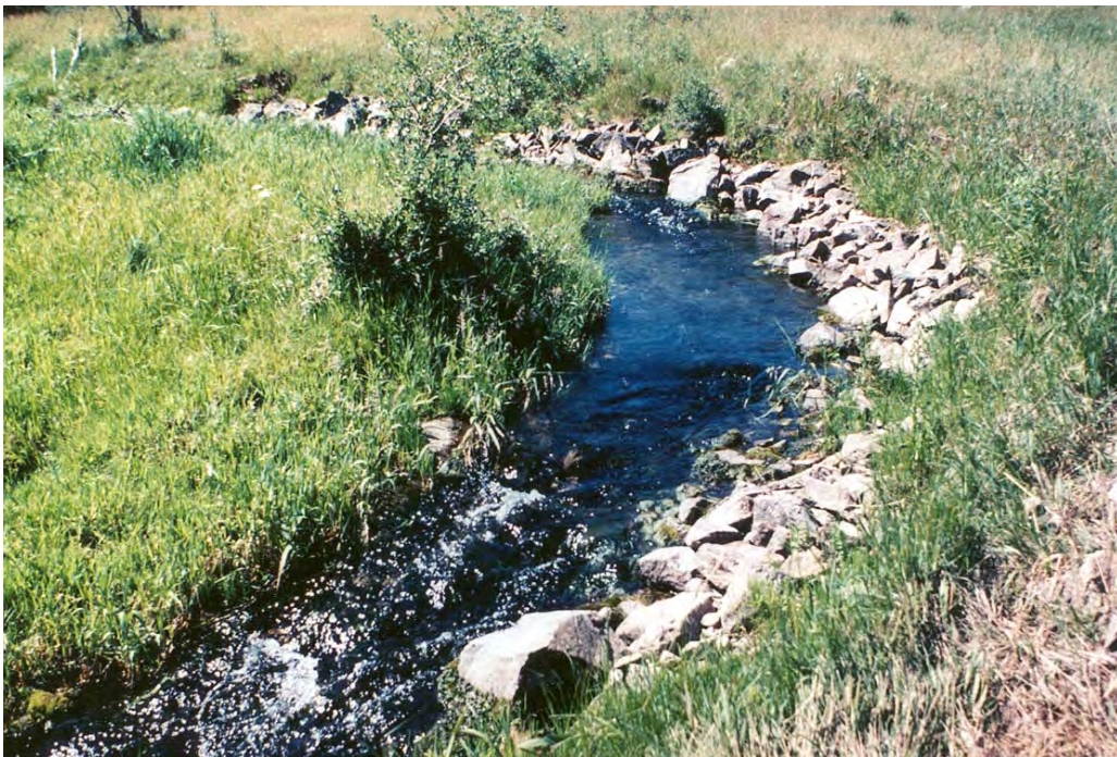
Figure 4-4. Eroding stream banks at Beaver Creek stabilized with rock riprap, which also sheltered trout by furnishing many hiding places among the rocks along the water's edge. Juvenile trout were especially fond of such habitat. Good vegetation growth and bank stability displayed at this site only two years after treatment.
