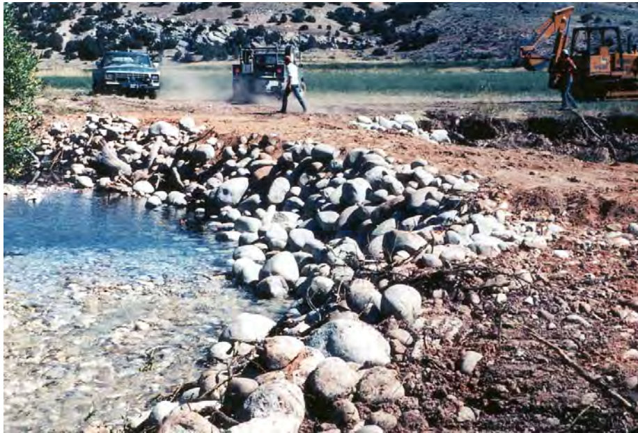
Figure 37-1. A 65 ft dike was constructed to divert all flow away from the channelized section and back into the old stream channel.
