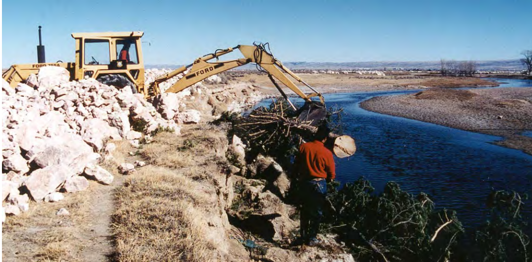
Figure 33-2. A WGF construction crew builds a tree/rock revetment. After the trees are placed, and anchored with cables to deadmen, the rocks are placed behind the trees to further anchor cable, trees, and bank. Note the point bars lack willows and other vegetation.
