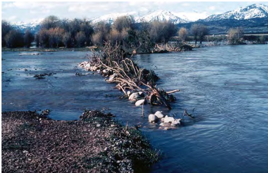
Figure 54-2. Due to the large volume of water and a degraded channel, spring snowmelt floods often flooded river bottom areas and threatened to cut through oxbows. Here a tree revetment is protecting a bank by reducing pressure on the bank from over bank flood flows.
