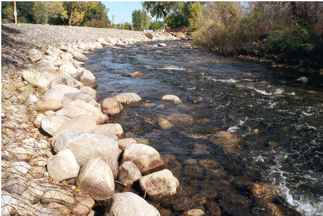
Figure 38-1. Stream banks through City Park had been treated years before by pushing river cobble up along the bank and covering the rocks with common stock fence. Subsequent corrosion of wire at river's edge allowed rocks to be sucked out from under the fencing by pressure differentials (Venturi effect) during high flows. Large boulders placed at the bottom of the riprap have successfully stabilized the banks.
