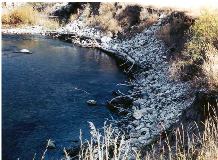
Figure 36-1. Addition of a tree/rock revetment to this steep bank during Phase I provided good overhead cover for trout along its base, stabilized the bank, and eliminated it as a source of sediment. Pretreatment, the river was actively eroding all along the base of the bluff, which contributed much sediment to the stream during high water.
