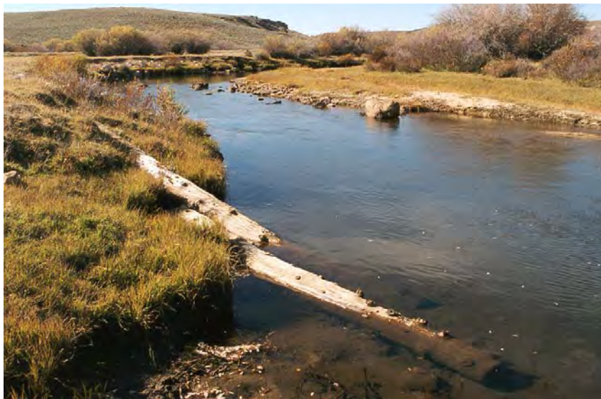
Figure 62-4. Two logs are all that remain of a log deflector installed 27 years previously. Attracting deflectors, like this one, were built to protect the bank on the left, but are still causing erosion (picture foreground, left). This type of structure is not
