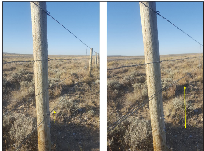
Figure 127. Installation of clips and ability to raise the bottom stand of the fencing.
