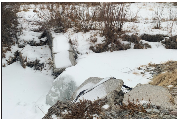
Figure 8. Dick Creek diversion dam. The dam continues to decline after the 2020 runoff and irrigation season.
