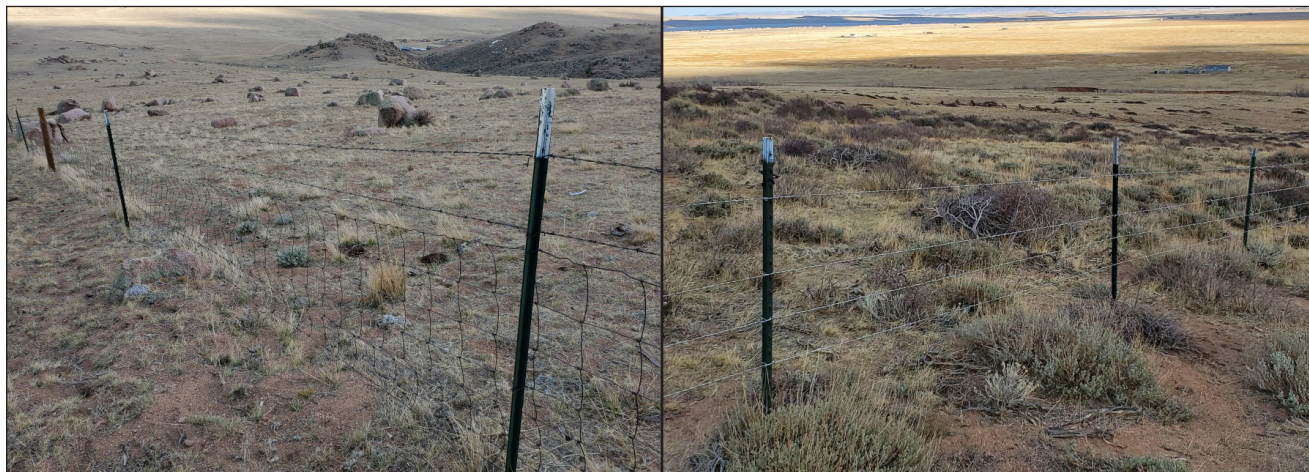
Figure 110. Fencing before (left) and after (right) conversion from woven wire/barbed wire to four-wire fencing.
