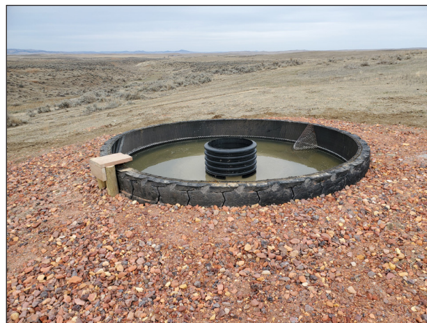
Figure 169. Installed livestock water tank.
