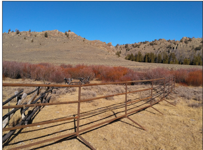
Figure 56. Steel jack replacement of old Palmer Draw exclosure fence near the confluence of Lander Creek and the Sweetwater River.
