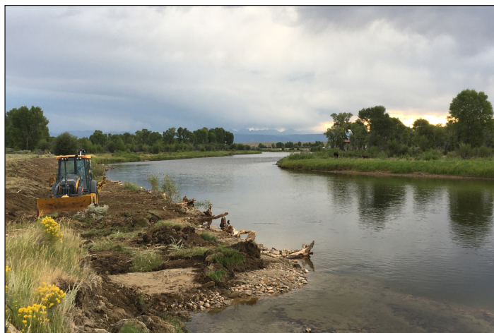
Figure 146. A bankfull bench being constructed on the Tatro Meander; a moose and calf look on at the new changes.
