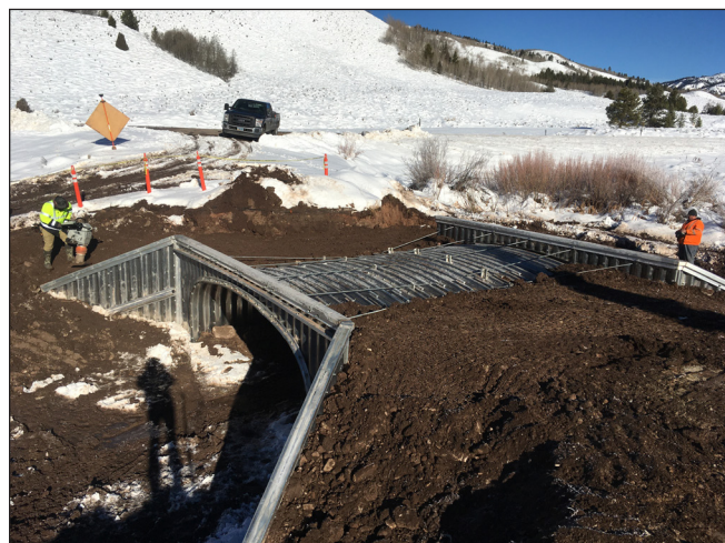
Figure 138. A new aluminum box culvert installed in Salt Creek to replace a perched and undersized culvert.
