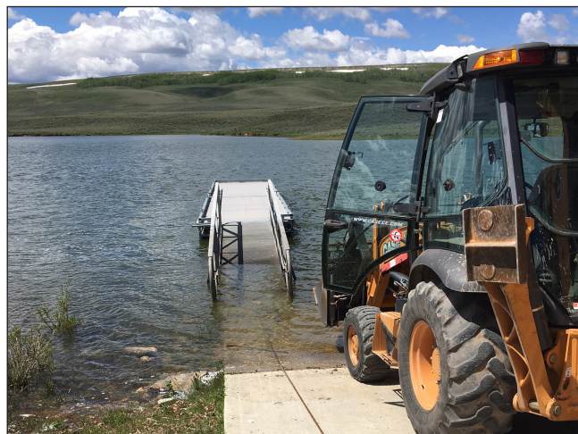
Figure 134. Resetting a boat dock due to seasonal weather fluctuations.
