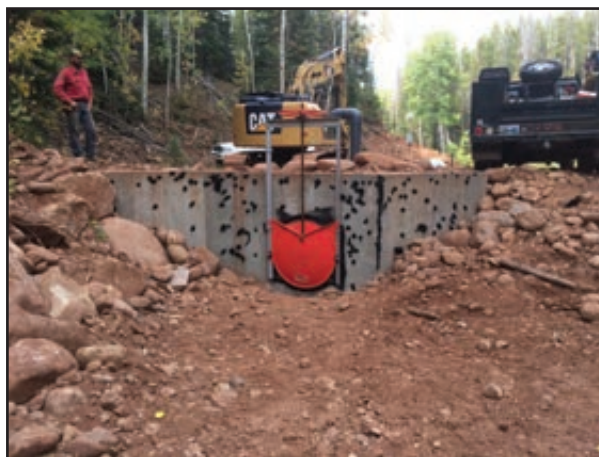
Figure 125. New dry wagonhound headgate.
