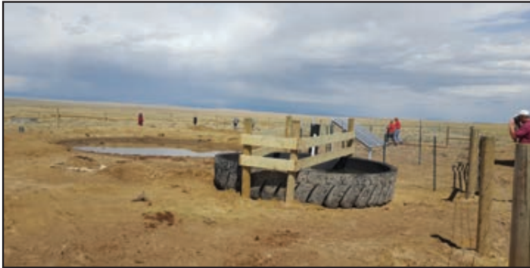
Figure 115. Installation day at the Ruby Knolls water development site in the Red Desert.
