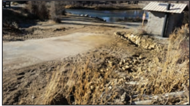
Figure 149. Access improvements to address parking drainage at New Fork Boulder Bridge PAA.
