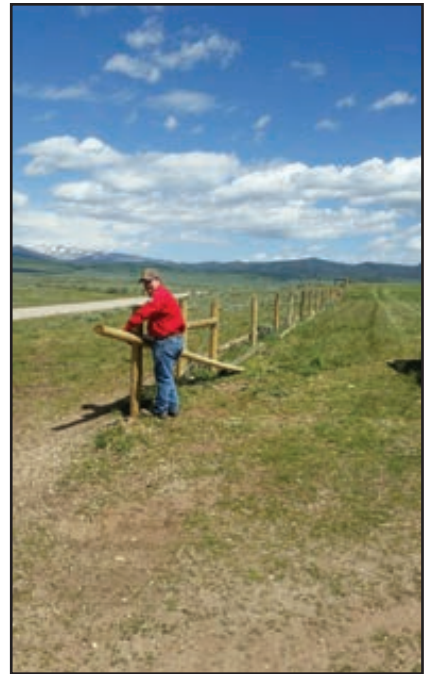
Figure 155. Construction of wildlife friendly pole top fence on the Black Butte WHMA.
