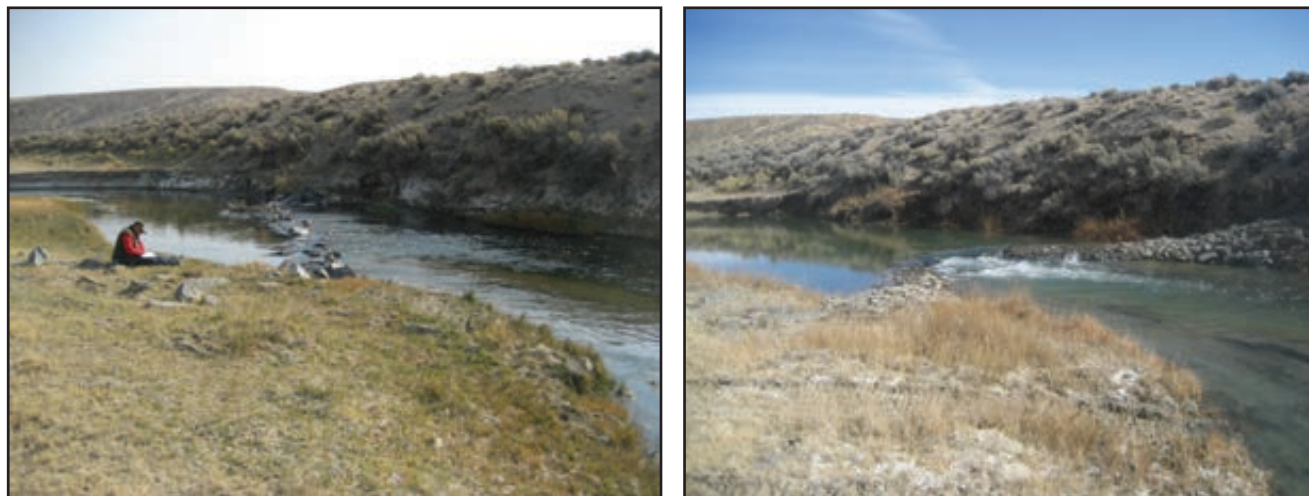
Figure 77. Before and after maintenance improvements to Sill #11 on the Lower Big Sandy River.
