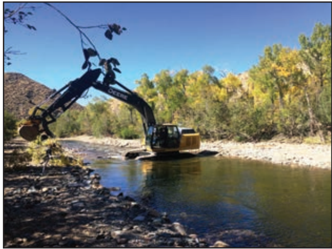
Figure 128. Constructing woody debris trout habitat cover in the newly shaped Encampment River channel at Oddfellows.
