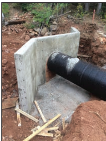
Figure 126. Heward pipe coming out of new headgate.
