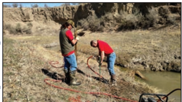
Figure 172. Department personnel planted cottonwood and willow cuttings at fenced buffers on Wild Horse Creek in Campbell County (top) and Beaver Creek in Weston County (bottom).
