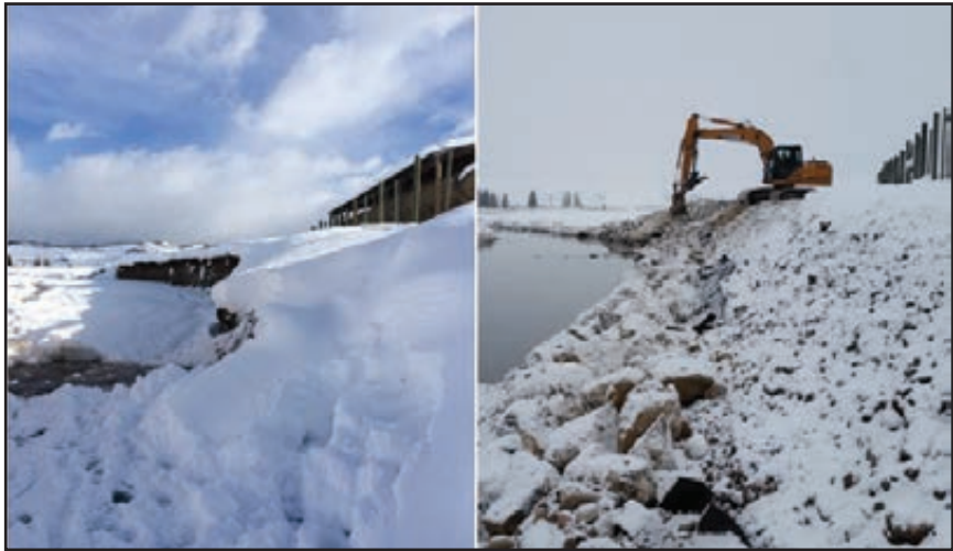
Figure 83. The McNeel bank stabilization site before (left) and after (right) installing a rock toe to protect the bank and feedground structures until a more permanent solution can be implemented.
