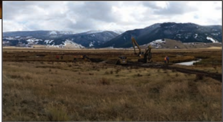
Figure 85. Tandem stream and riparian exclosure fence construction on Flat Creek during October 2016.
