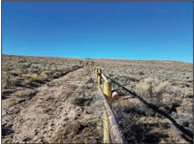
Figure 118. Fence was converted to a wood post/rail top design with two barbed and one smooth wire to improve wildlife movement and hold up to cattle/wild horse pressure. Photo courtesy of BLM.
