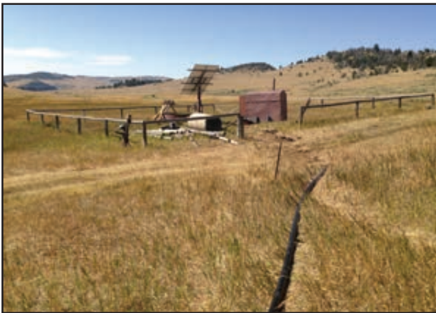
Figure 188. Upgraded solar well setup and distribution lines.
