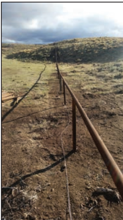
Figure 154. Partially constructed wildlife friendly drill stem pipe fence surrounding Fall Creek WHMA.
