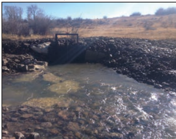
Figure 72. New headgate and rock vane installed to improve water delivery and fish passage. Photo courtesy of TU.
