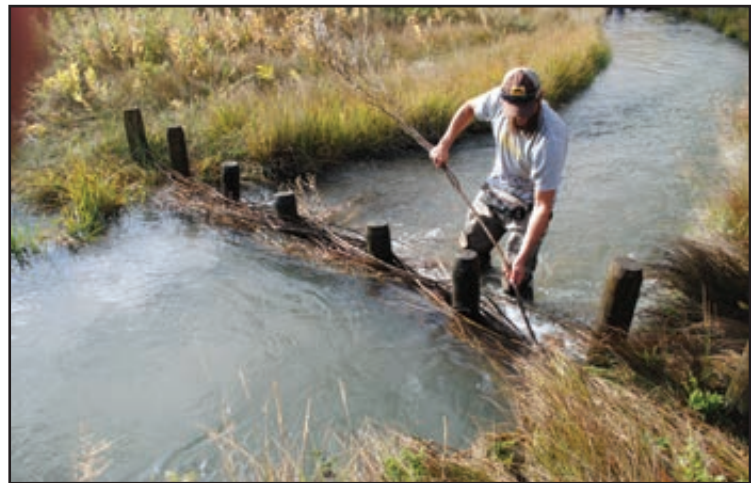
Figure 49. Constructing a beaver dam analogue.
