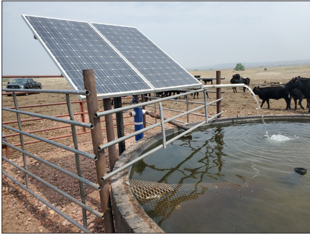
Figure 157. Livestock stock tank with a solar well installed to improve livestock grazing distribution.
