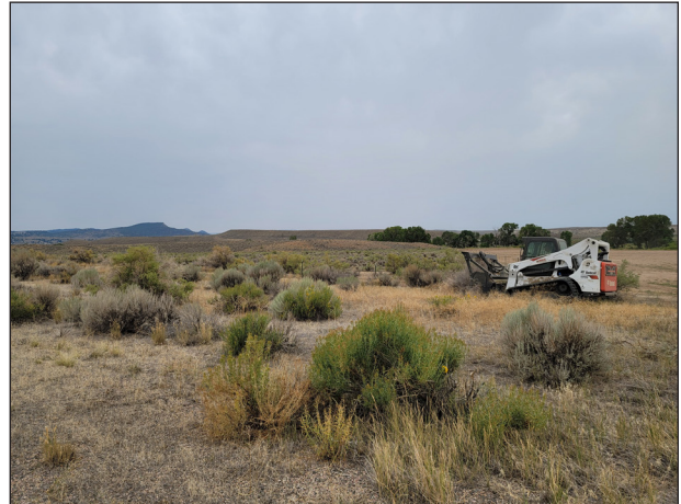
Figure 1. Shrub treatment along Highway 487 to reduce mule deer concealment cover and prevent deer-vehicle collisions.
