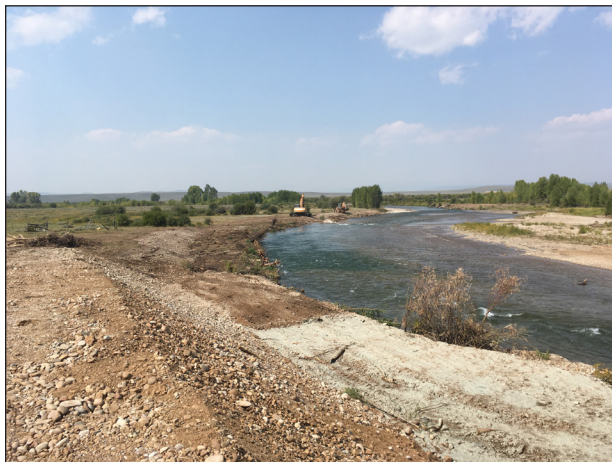
Figure 115. Construction of a bankfull bench with toewood at the Daniel Access Area.
