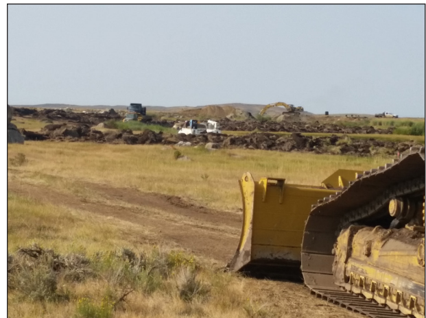
Figure 129. Dam construction and install of final structure on Soda Lake Wetland pond.
