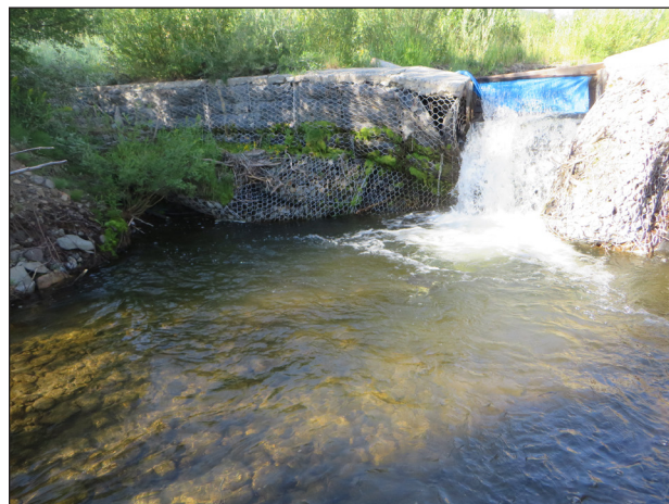
Figure 26. Sunshine WHMA failing diversion on Dick Creek.
