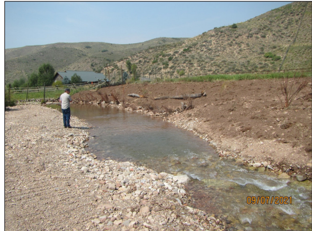
Figure 54. Contractor inspects the newly constructed bankfull bench, rock and log toe, and rock J-hook at the WGFD Horse Creek WHMA.
