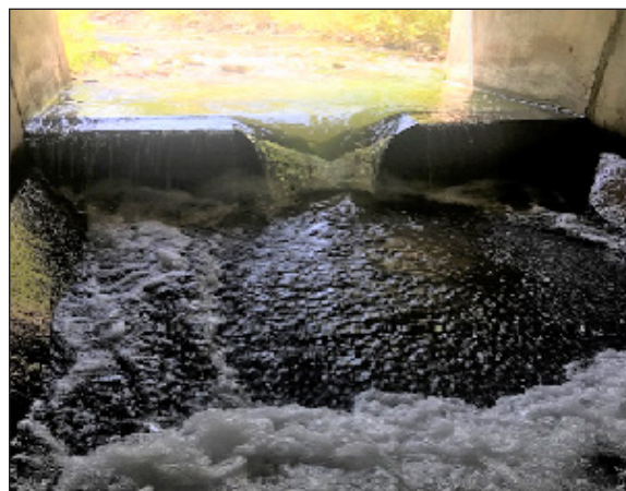
Figure 61. Cabin Creek, the highest passage priority in Teton County, features an undersized concrete culvert.
